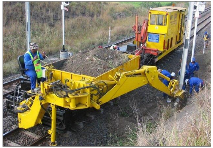
Utility Vehicle with Drain Cleaner
